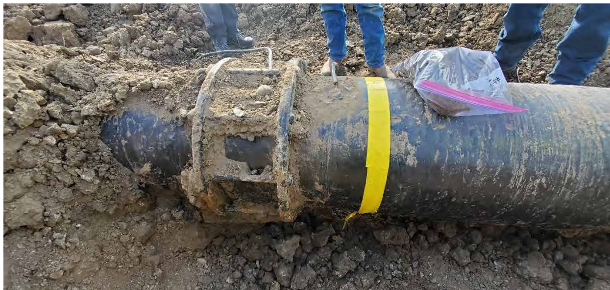
Figure 3 – Pipe and Coupling Conditions
