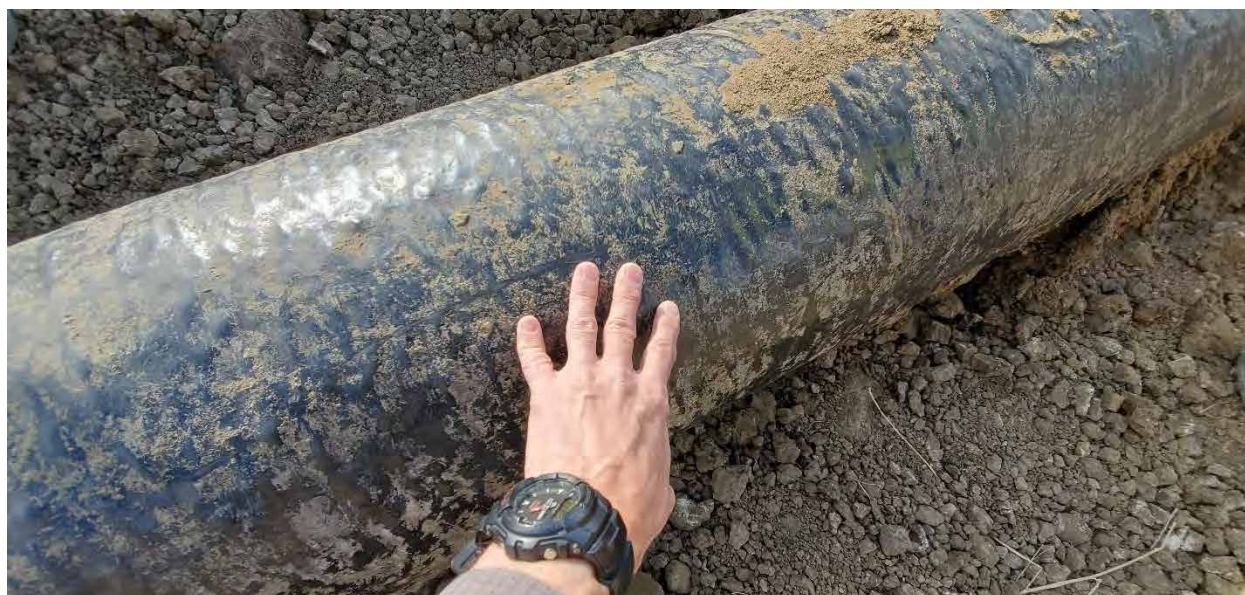
Figure 4 – Pipe Coating Conditions
